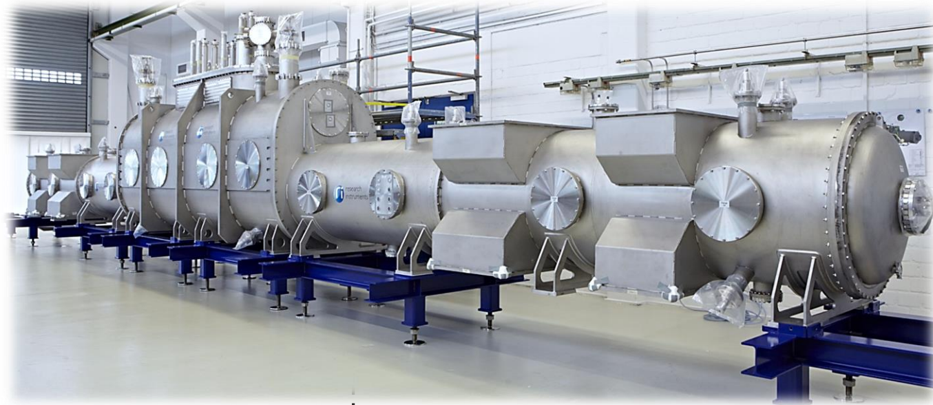
Windowless Gaseous Tritium Source cryostat
