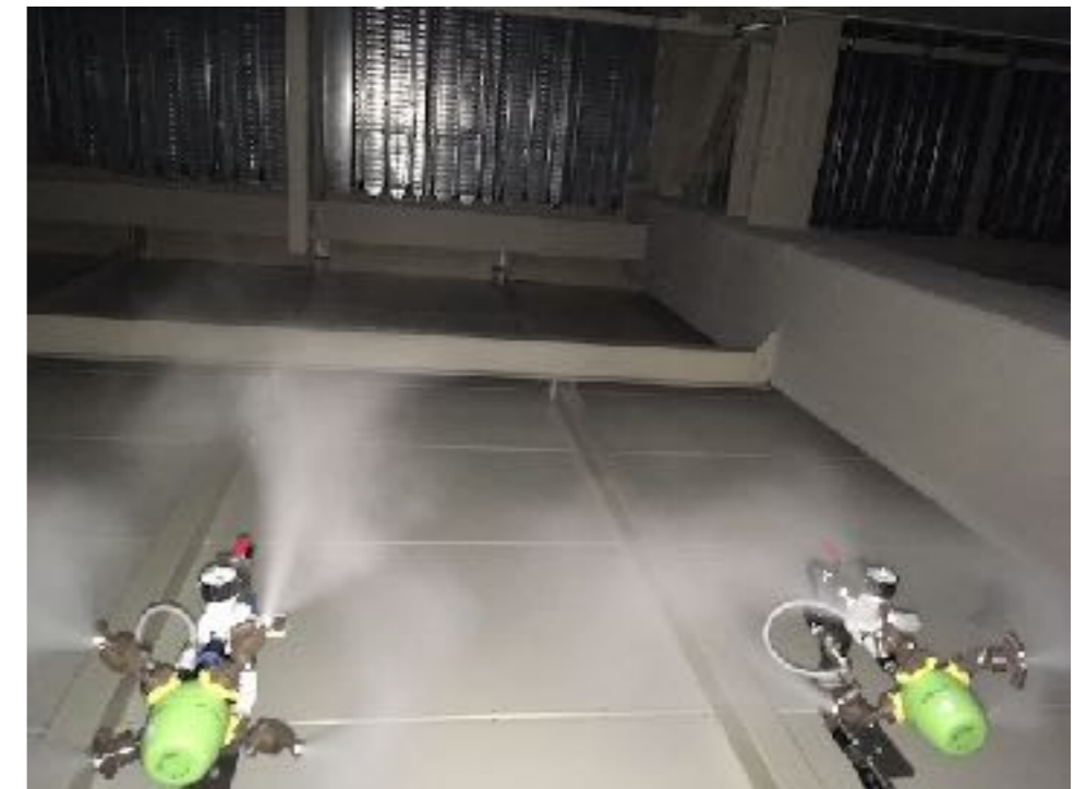
Mist generation system just before ULPA (HEPA) filter
